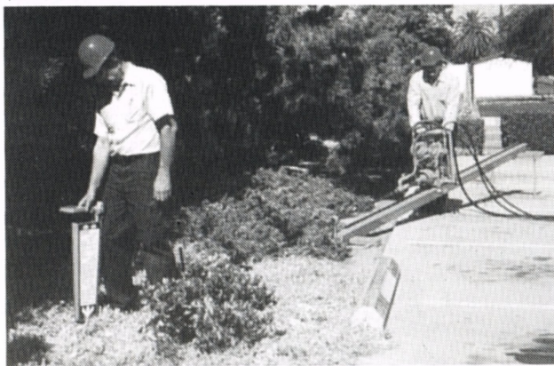
The Directional Boring Machine in operation. In the foreground is the hand held drilling bit locator showing the location and precise depth of the boring head.
