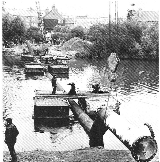
690mm (27") dia. steel pipe being floated into position across the River Trent at Burton.
