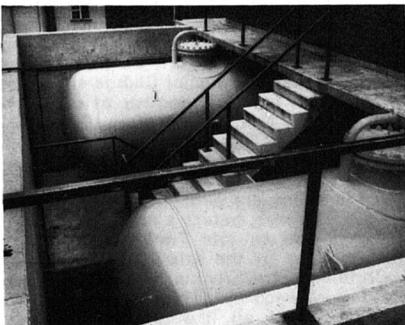
The Chlorine Storage Tanks.
